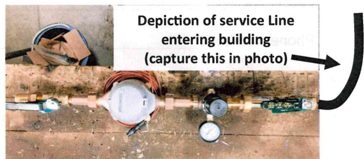
Example of a typical water meter assembly
