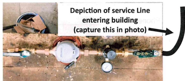
Example of a typical water meter assembly
